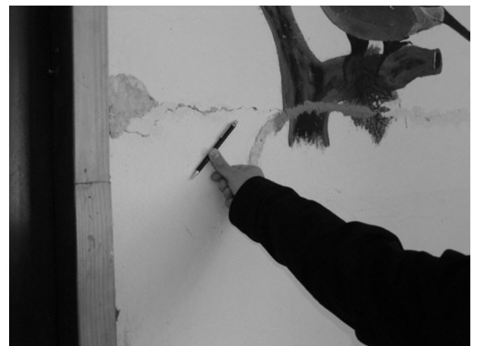
Figure 7: Cracks in the wall of a house in Reinaldo Espinosa area
