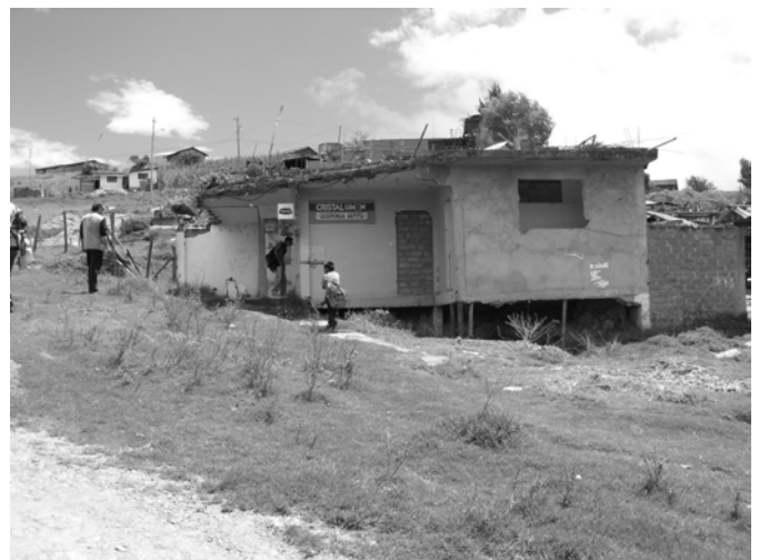
Figure 6: Damaged House in Reinaldo Espinosa area
